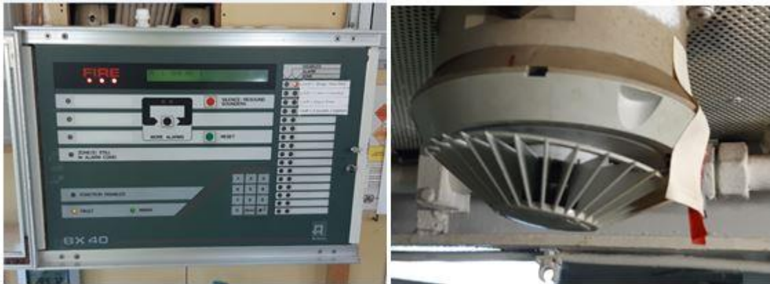
Figure 38 Fire detection system – main panel and engine room detector head.
