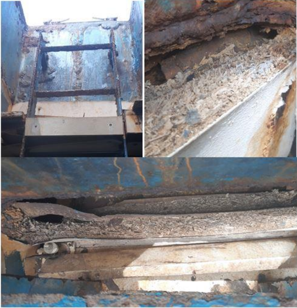
Figure 16 Corrosion in way of forward focsle hatch access from sleeping quarters.
