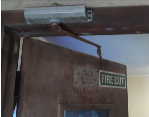
Figure 27 Hatch to engine room does not appear to be A-60 rated.
