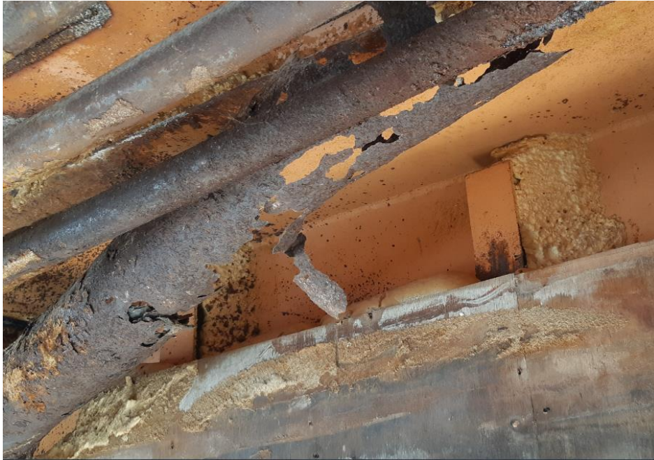
Figure 25 Corroded piping in cargo hold that leads to engine room ventilation.
