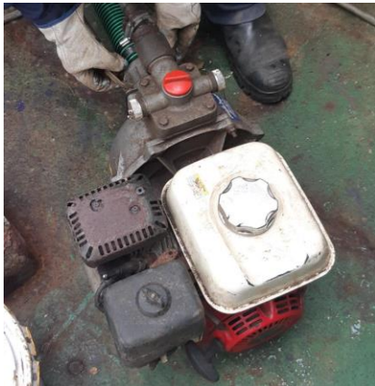
Figure 5 Emergency fire pump.
