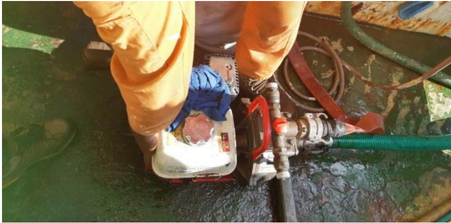
Figure 23 Emergency fire pump.
