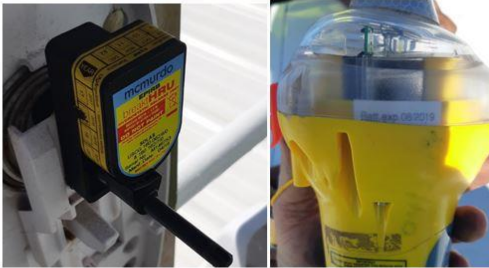
Figure 43 EPIRB Battery and release unit expired.
