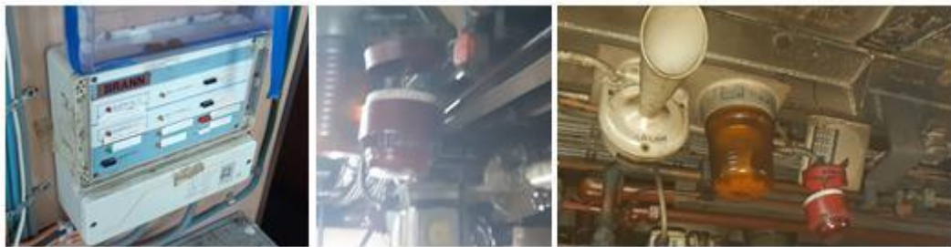
Figure 4 Fire Detection System.
