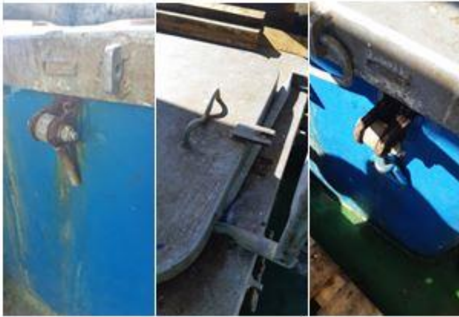
Figure 20 Smaller hatches (aft) missing securing cleats / dogs. Forepeak sounding pipe securing cleats broken. A number of doors with stiff dogs noted and electrical cords passed through.
