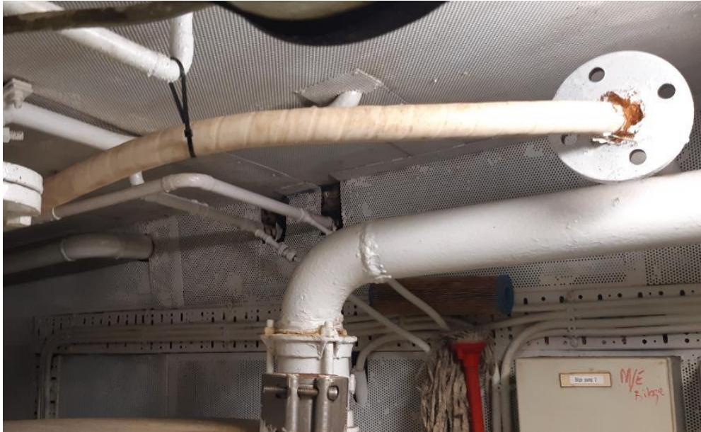
Figure 46 Sewage holding tank bypass for lower decks.
