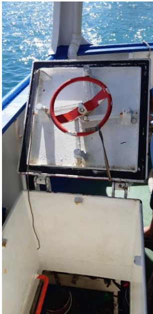
Figure 37 Aft hatch to steering gear not sealing – note this also has access to engine room which is typically not secured. Flooding into this space could also flood engine room.
