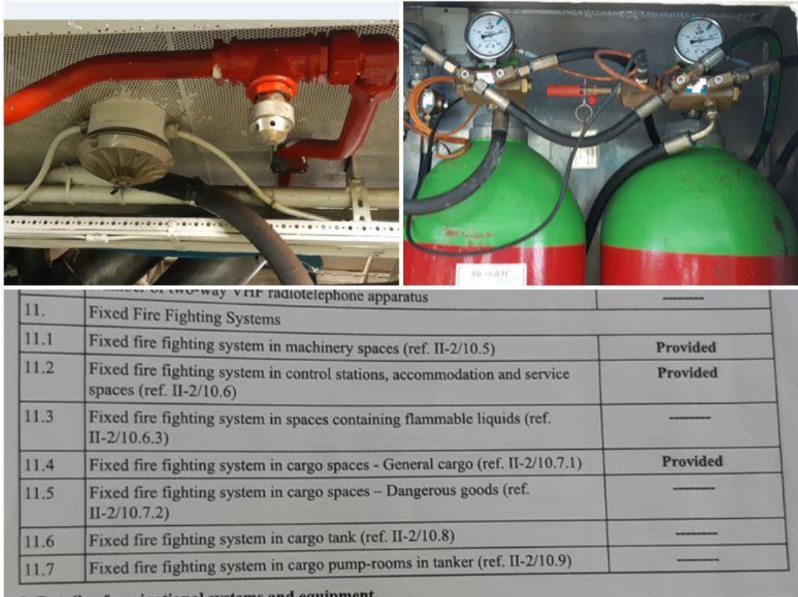
Figure 39 Fire Suppression System and Safety Equipment Certificate.
