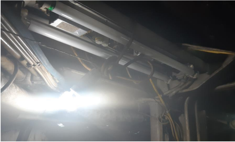
Figure 15 Lighting in engine room is broken. Power cords run to extra lights. This is unsuitable as doors cannot be closed fully to prevent fire. Demonstration of poor maintenance.
