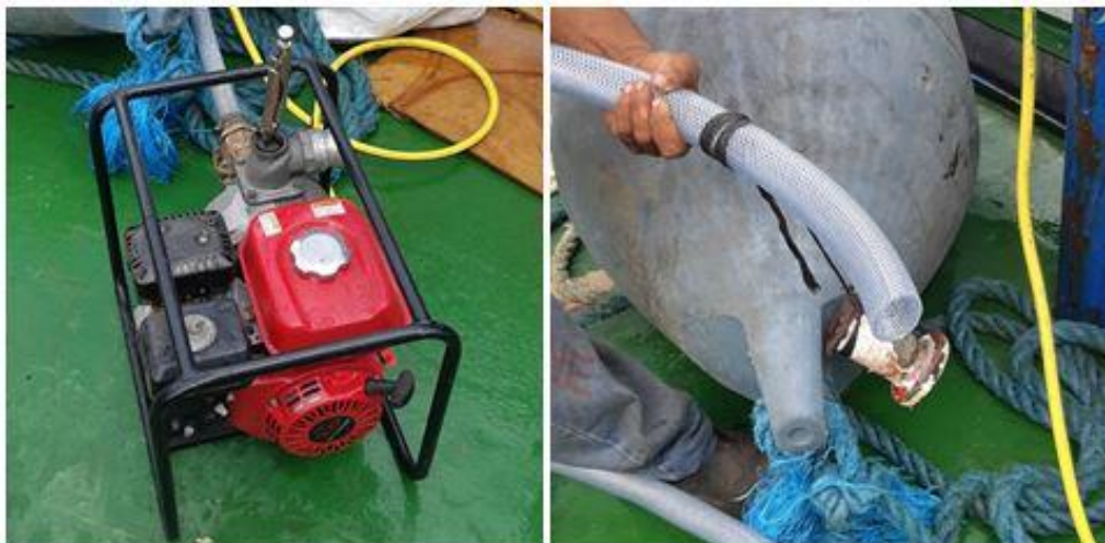
Figure 40 Emergency fire pump.
