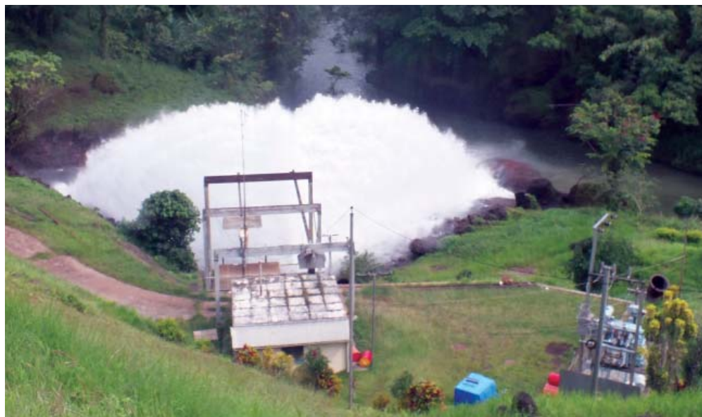
ADB helps Pacific DMCs to develop and manage their hydroelectric potential—a valuable indigenous resource
